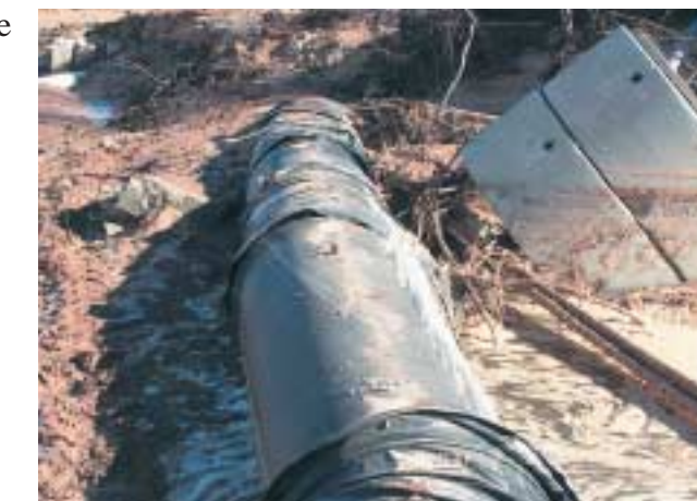
Regional Pipeline Exposed at Johnson Diversion
