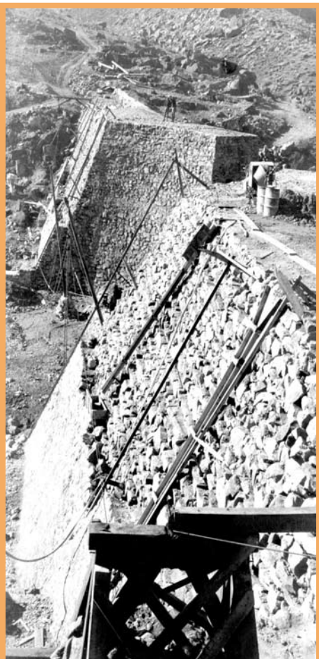
Winsor Dam receiving a coat of veneer on its downstream face by C.C.C. workers — 01/01/1935
