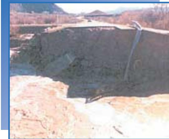
Bridge on River Road was washed out. The car is headed to Bloomington Hills; the road veering off to the left runs under Stone Cliff toward the Springs subdivision.* (1966)
